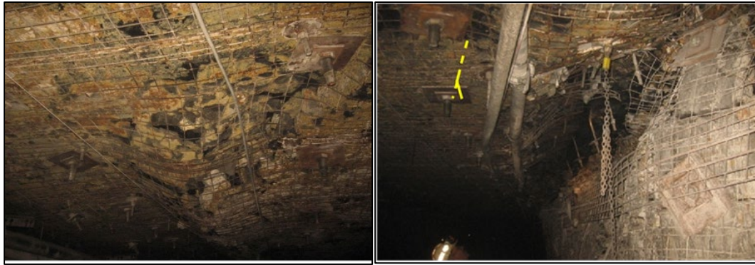
Figure 24. Austar gateroad centreline bagging and chain pillar side guttering near bent tendons (Moodie, 2011)
