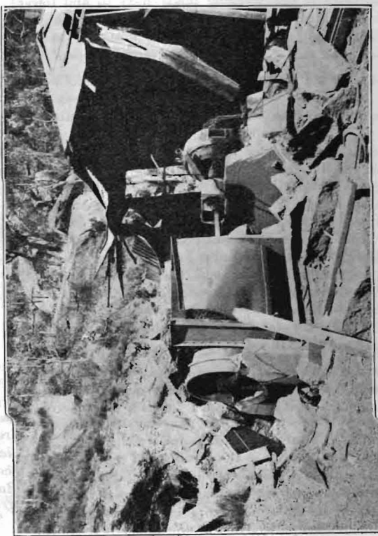
WRECK OF THE EXHAUST FAN, AT OUTLET OF THE FAN TUNNEL.
